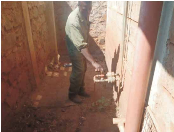
Photo 2.6: Close all peripheral valves of the block and all the customer valves completely
