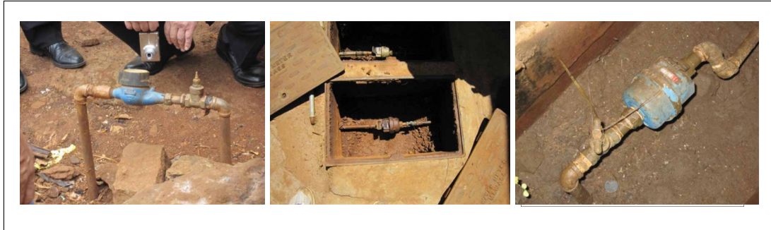
Photo 2.4: Customer Water Meters in Embu
