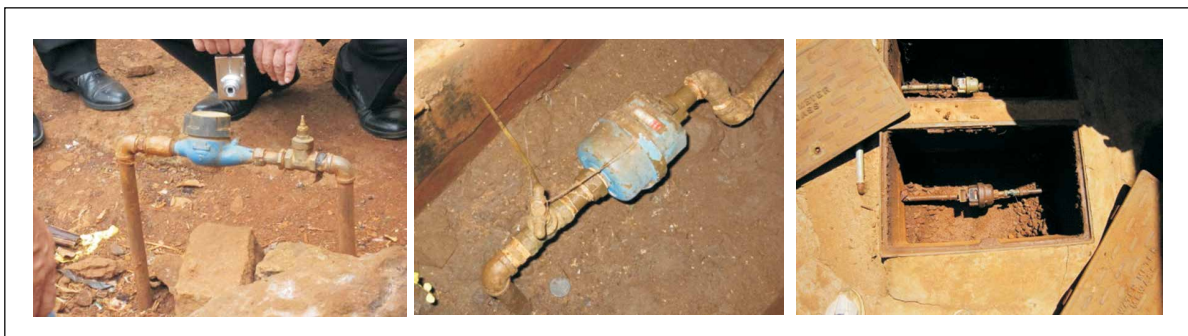
Photo 4.2, 4.3, 4.4: Example of Water meter
