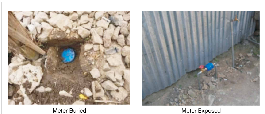
Photo 4.1 Buried and exposed customer meter
