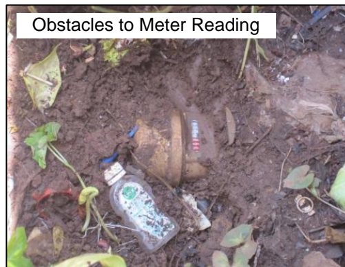
Figure 6.7: Water Meter Covered in Mud
