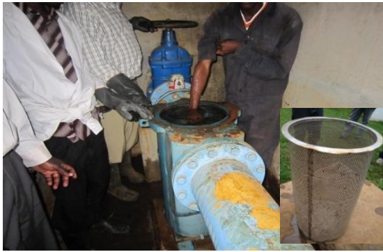
Figure 6.1: Strainer (Installed at outlet of Water Treatment Plant) (Meru WSP)
