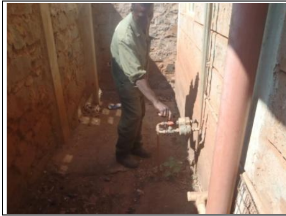
Figure 8.5: Close all peripheral valves of the block and all the customer valves completely
