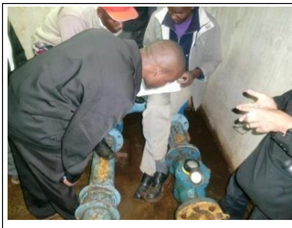
Figure 9.8: Flow Meter Reading
