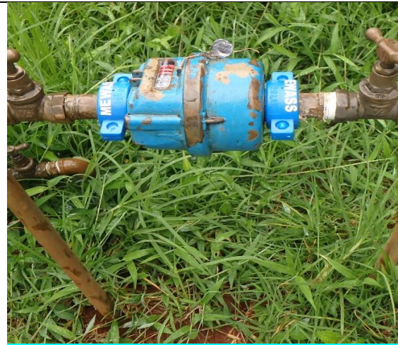
Fig. 8.12: Meter Sealed Using Plastic Seals
