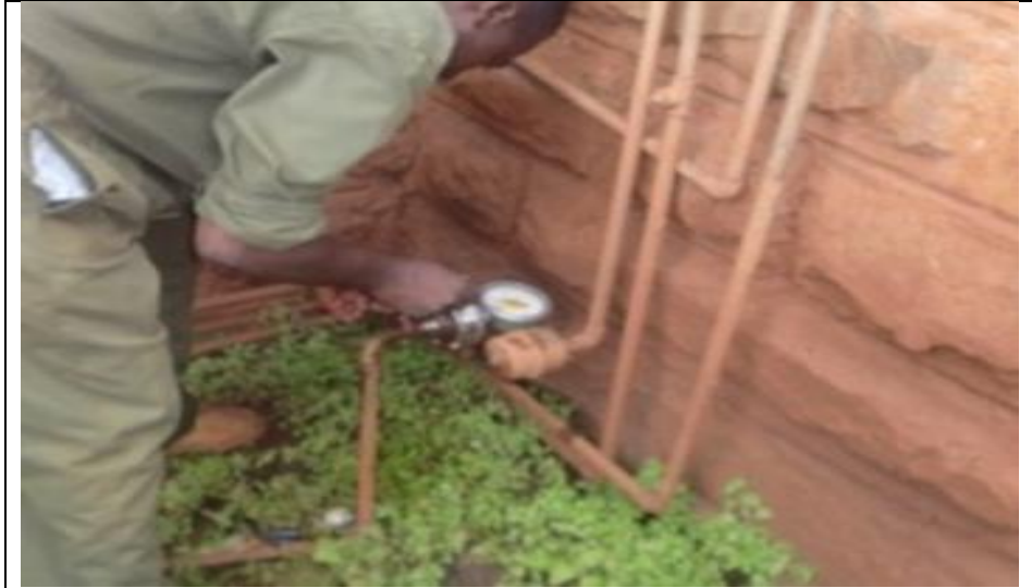
Fig. 6.3: Pressure gauge installed at customer metering point
