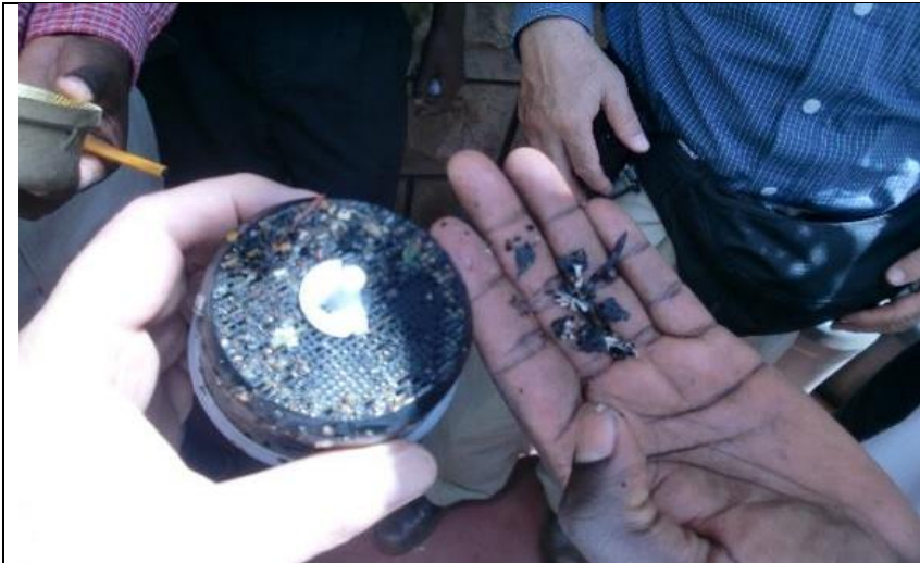
Fig. 8.3: Debris trapped meter strainer
