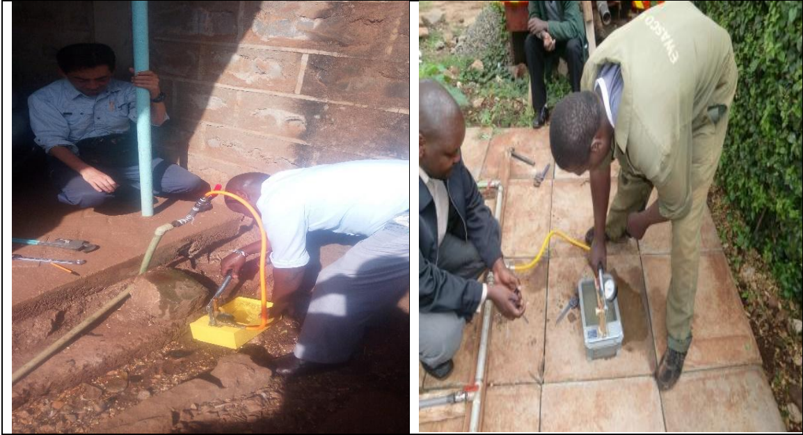
Fig. 7.1: Handpump connected on different pipe materials ready for use
