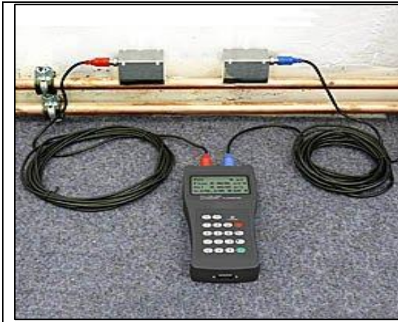
Fig. 5.9: UFM mounted on pipe
