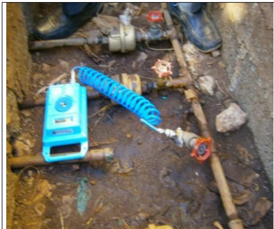
Fig. 6.6: Pressure Logger Installed on Pipe
