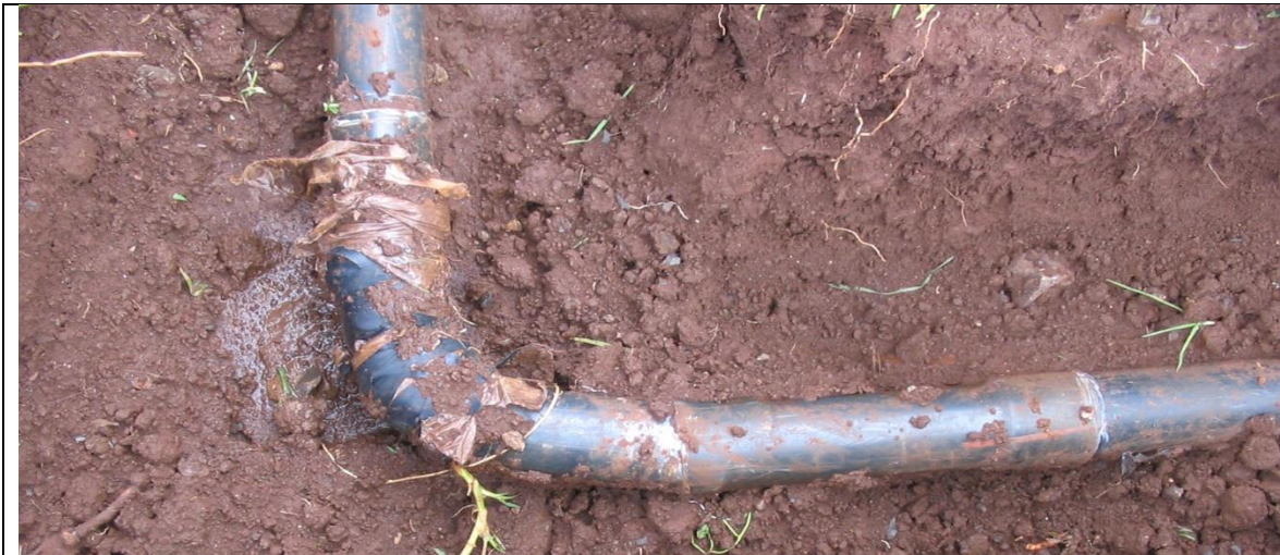
Fig. 2.15: Poor Repairs with Fire Couplings
