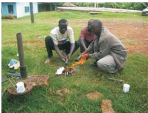
Photo 7.1: Fire Coupling (used for pipe connections in Kenya)
