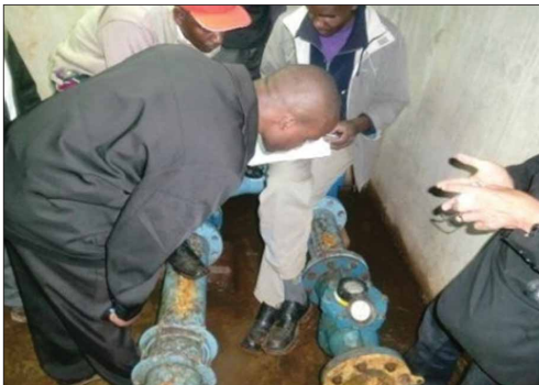
Photo 3.6: Flow Meter Reading
