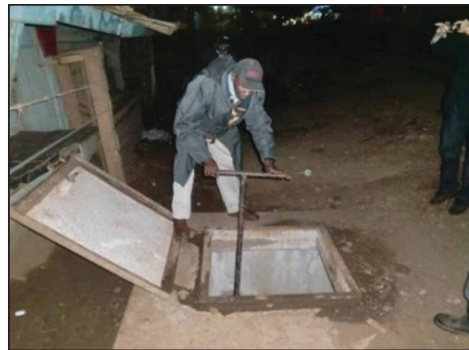
Photo 3.7: Closing Gate Valve
