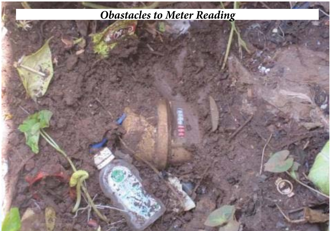
Figure 6.7: Water Meter Covered in Mud
