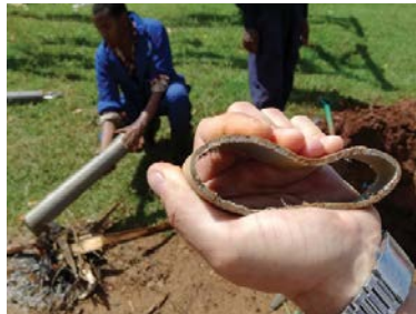
Figure 8.9: Degradation of pipe caused by excessive heat on the UPVC pipe.
